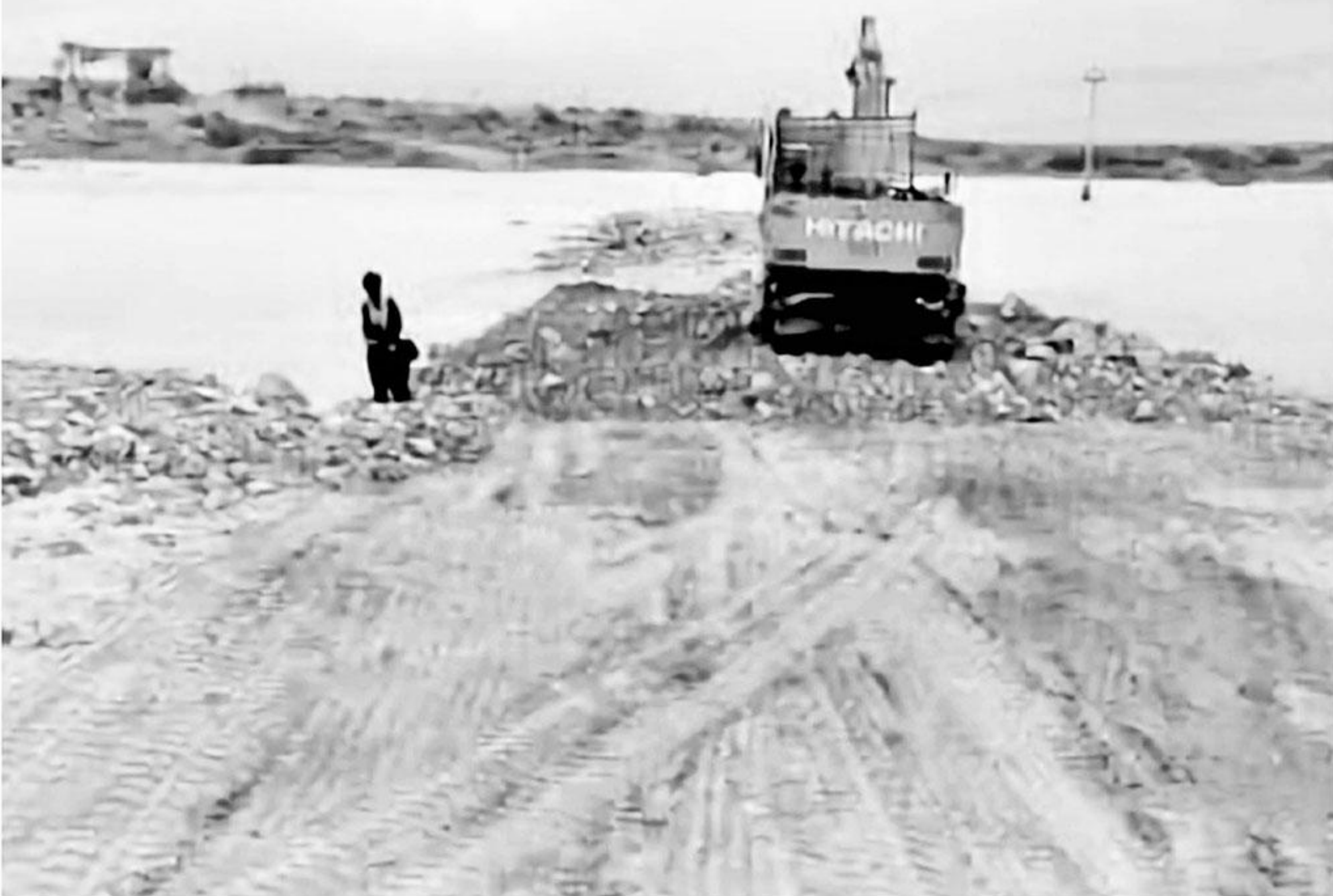
HUB: The construction work of causeway crossing road that was completely destroyed by floods is underway here on Monday. —PPI photo
